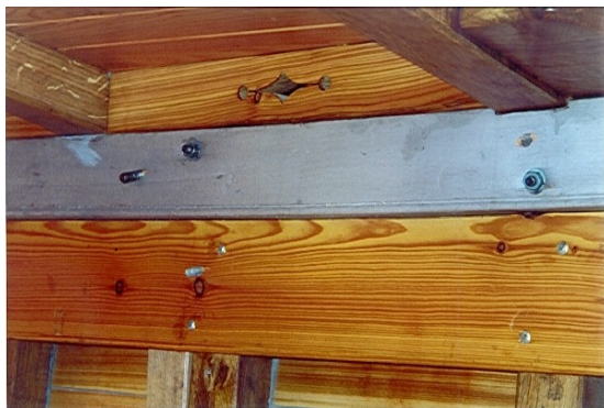
Note the attention to detail he has given to the air vents to the cover boards
